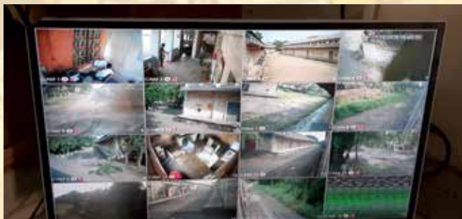
CCTV surveillance system at warehouses of Central Warehousing Corporation
